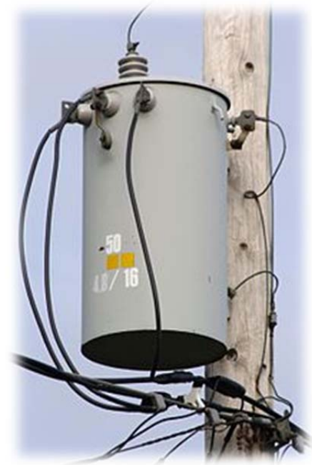
Pole-mounted distribution transformer with center-tapped secondary winding used to provide 'split-phase' power for residential and light commercial service, which in North America is typically rated 120/240 volt.
